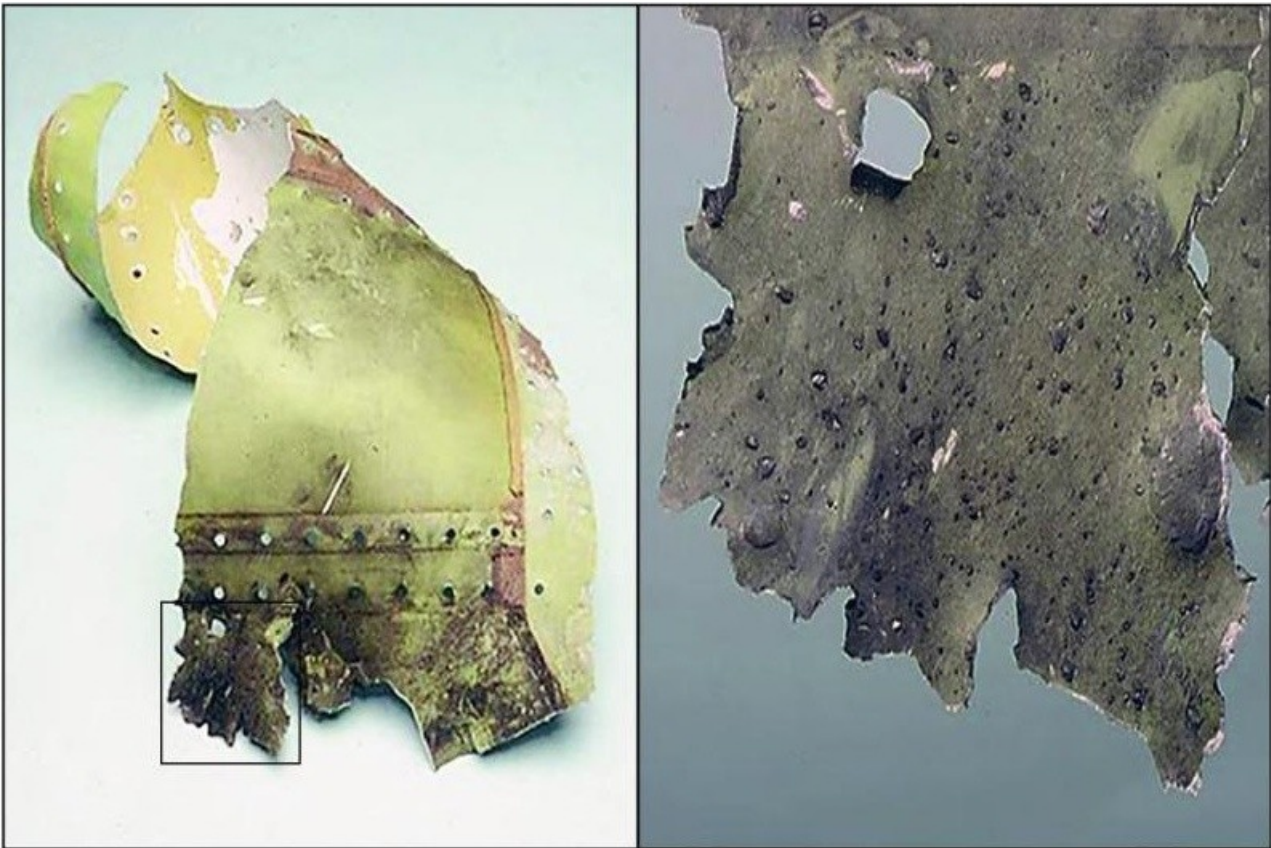
Fig 2: A concentration of staining and microcraters with some gas wash near the tip of a curl from a petaled hole torn in an aircraft fuselage by explosion. No such marks have been found in Smolensk. (Source: Forensic Investigation of Explosions , CRC Press, © J. Garstang)
